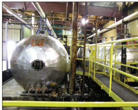
The visit includes a look at one of the newly installed treating cylinders.
